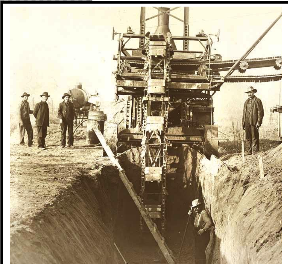
Crews use a trenching machine to install a 48-inch wood stave pipe near Alameda Avenue in this November 1909 photo.
