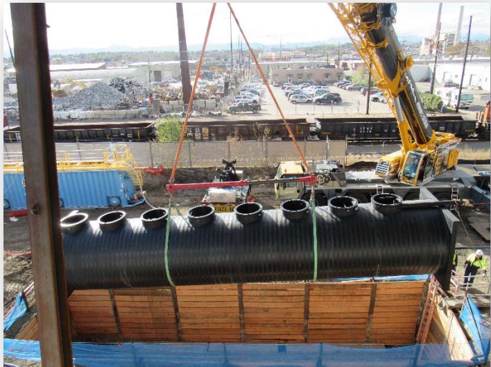
The multistage treatment unit (MSTU tank) on the west side of the Administration Building is one component of the Wastewater Recycling System as part of the overall One Water strategy of the complex redevelopment.
