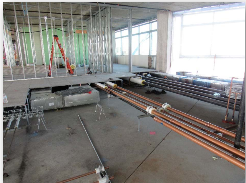
Raised flooring and radiant heating in the Administration Building
